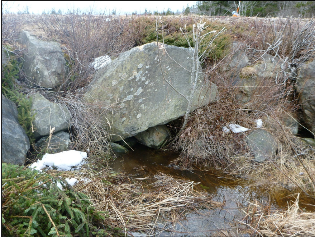
Figure 7 Culvert upstream: partial blockage by armour stone (24 February 2014).
